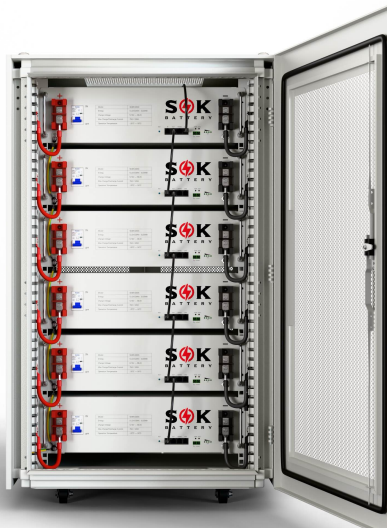
30kWh 6 x SOK Rack Batteries
