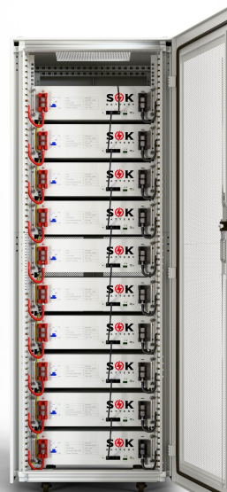
50kWh 10 x SOK Rack Batteries
